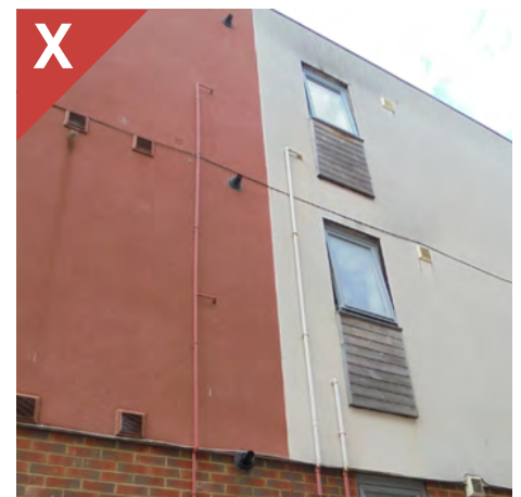
Figure 2.27c: Flues, vents and pipes add clutter to the façade.
