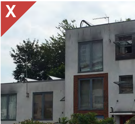
Figure 2.23h: Use of render that weathers poorly and not be maintained.
