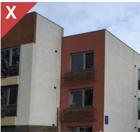
Figure 2.23j: The change in render colour at the corner contributes to a flimsy appearance, highlighting that it is surface applied and lacks depth.
